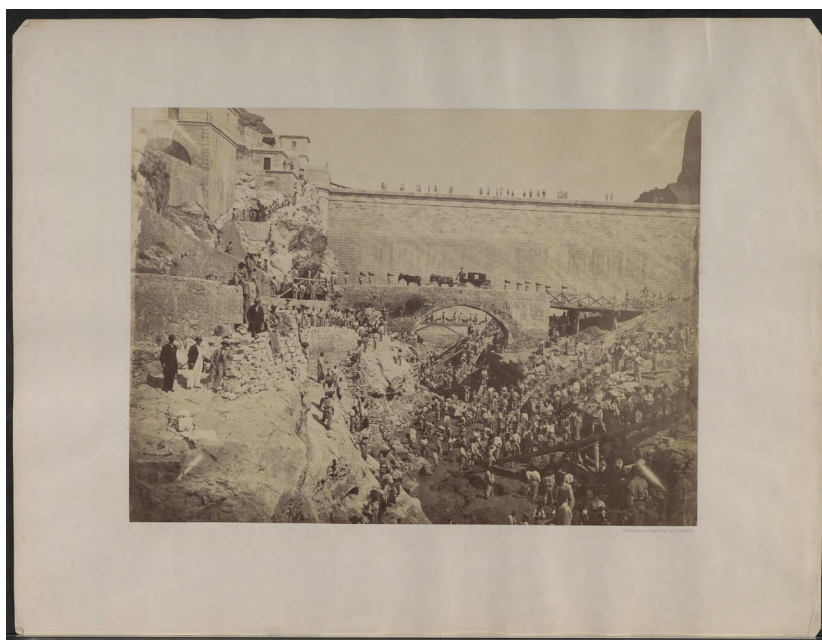
Fig. 1: Worksite of the dam Pontón de la Oliva for the Canal de Isabel II in Madrid in the 1850s taken by Welsh photographer Charles Clifford (ca. 1850s), Biblioteca Nacional de España, http://bdh-rd.bne.es/viewer.vm?id=bdh0000258154 .
