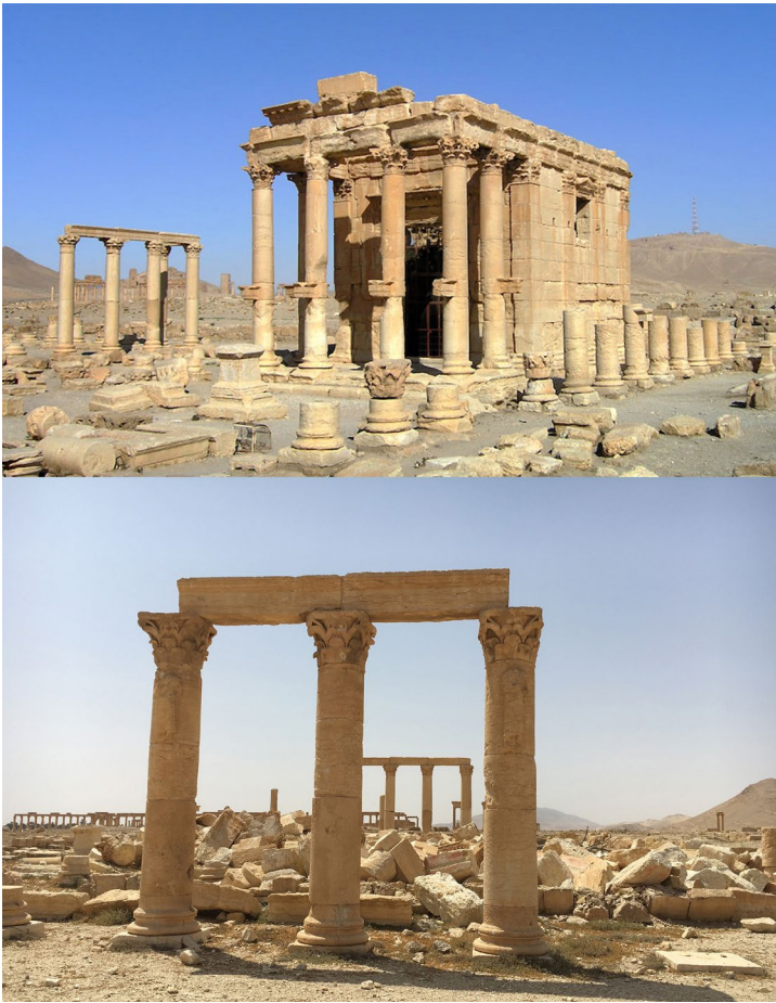
Fig. 2.4 Temple of Baal-Shamin. Damage assessment of Palmyra. Photographs by DGAM, 2017, CC BY-NC-ND.
